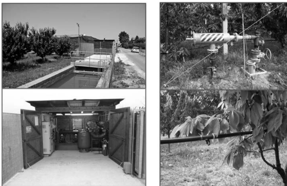
Figure 2 - Diamante Plant – pumping station and pipe lines
