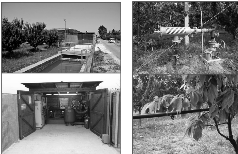
Figure 2 - Diamante Plant – pumping station and pipe lines
